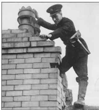
Fireman Dave Jones removes dangerous loose brick from a chimney stack in Silverlea Avenue, Wallasey after a storm
